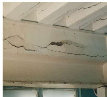
Cracks in wall and roof at Port Royal Police Station.
