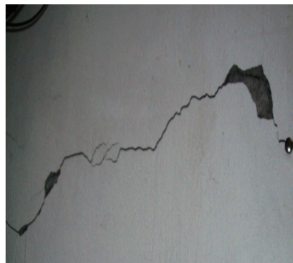
Crack in wall at Rockfort Police Station.
