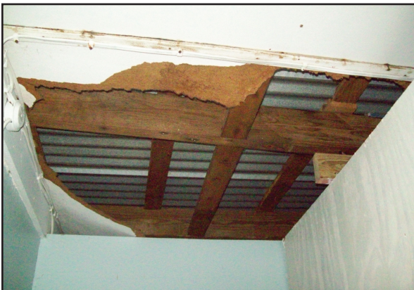
Photo 5: A damaged section of the ceiling at the Retreat Station as presented on 29/10/2012.
