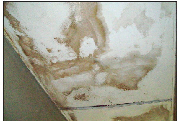
Photo 6: A water damaged section of the ceiling at the Highgate Station as presented on 30/10/2012.
