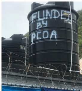
Water tank installed at the Bull Bay Station in the Kingston Eastern Division.
